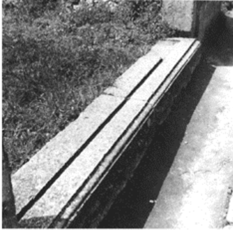
730 Entrance to a shop at Pompeii (VII, 12, 11), showing the groove for fixing the shutter in front of the counter; note also the passage left for the door at one end.
