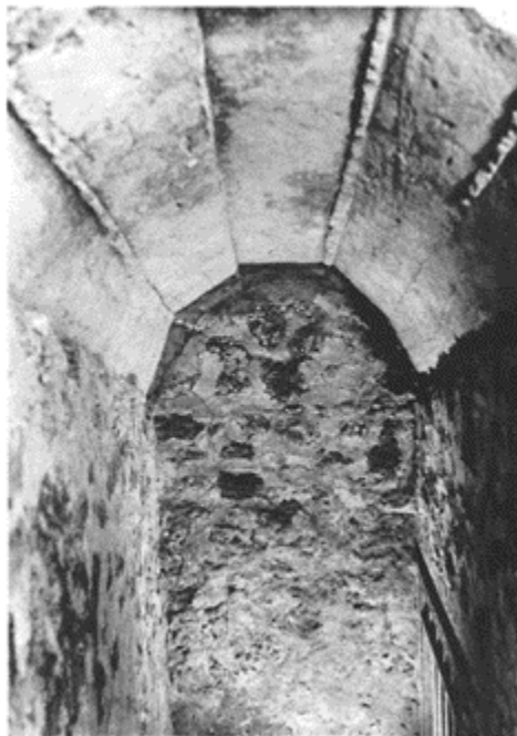
432 An imprint of centring made of wide planks (25 to 30cm) in the arch of a staircase in the Villa of the Mysteries.
