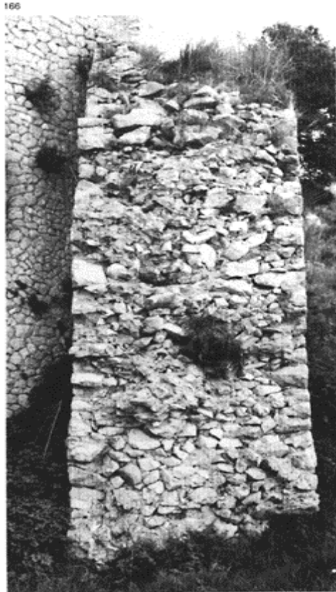
166 Cross-section through masonry of the Later Republican period (walls of Terracina, dating to between 100 and 90BC) with facings of opus incertum and rubble core. Note the horizontal
