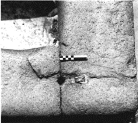
598 Detail of the jointing of two dressed stone slabs in the trough of a public fountain at Pompeii, showing the channel into which was poured the string-course of mortar for
