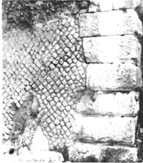
305 The amphitheatre of Cassino ( Casinum ) (late first century BC), with a facing of opus quasi-reticulatum with quoins of ashlar construction.
