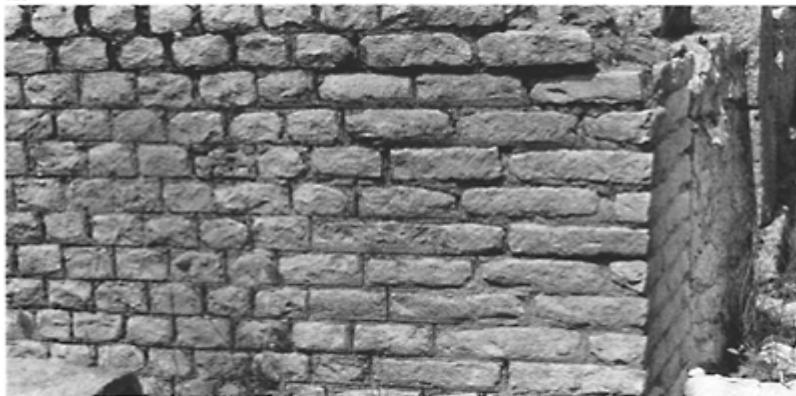
325 Wall of 'petit appareil' at the Theatre of Argentomagus (St-Marcel). The stones of the quoins have been made larger so as to have a greater contact surface with the masonry and so give more cohesion to this section.
