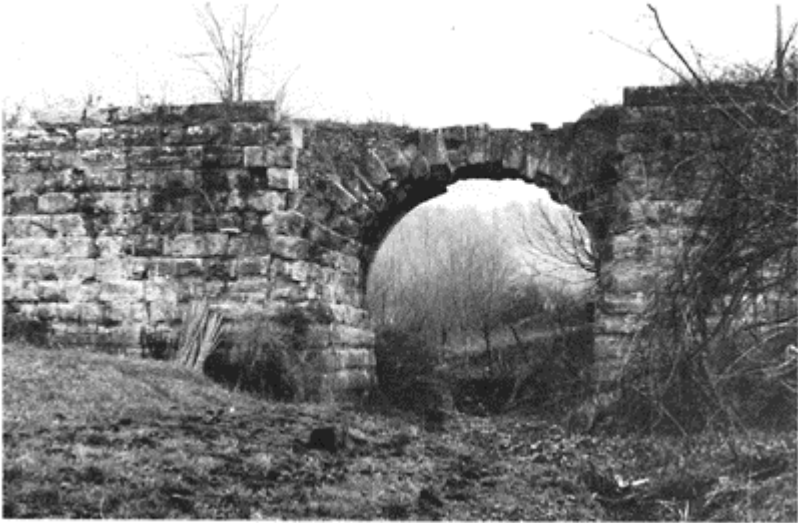
658 The Ponte Amato, on the via Praenestina , below Gallicano. On each side of this single-arched bridge is a large stone mass to avoid a fall in the level of the roadway.
