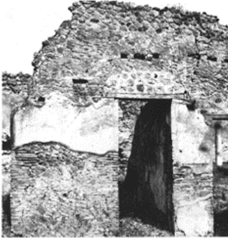
365 Pompeii, reconstruction after the earthquake of 62. Wall made up of varied terracotta material: bricks, tiles, fragments of amphorae (IX, 6, 3).
