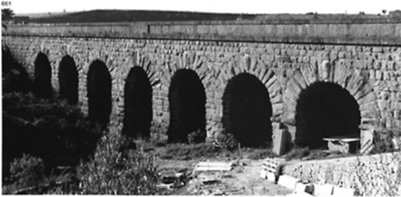
661 The Ponte di Nona on the via Praenestina at the ninth mile after leaving Rome. Length: 125m; height: 16m; c. 100BC.
