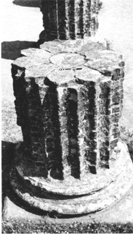
370 Brick column from the Basilica of Pompeii. Around a central cylinder are arranged the 'petals' forming the fluting; a stucco rendering covered the facing.
