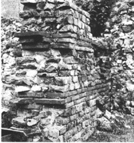
340 Wall of 'petit appareil' with brick courses joining the two facings, at the Forum of Bavay. Second century.
