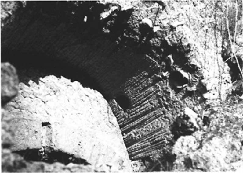
434 The traces of reed formwork covering the centring, used in the construction of a masonry vault. Pompeii, I, 3, 31.
