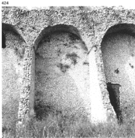
424 A section of the niche arches of a terrace at the temple of Fortune at
