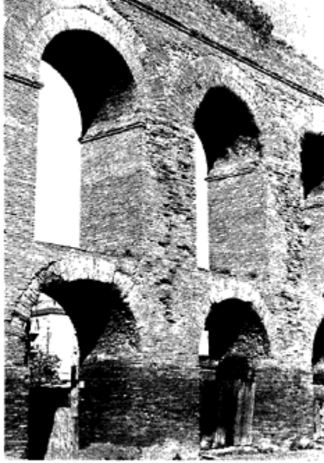
430 Arches of the aqua Alexandriana , one of the aqueducts of Rome. The upper arches, bearing the weight, are faced at the crown with two rows of bricks; the lower braces have only one; c. 226.
