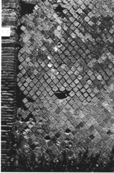
188 Wall of reticulate construction, in which can be seen the putlog holes of two levels of scaffolding, each with a small lintel. Pompeii VIII, 2, 30; c. 70.
