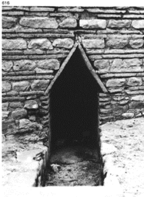
616 The outflow from the Baths of Velia. The bricks or tiles serve as corbelled centring in the masonry.
