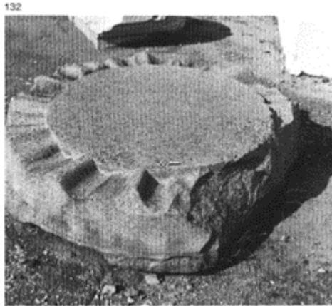
132 Wavy joint in a granite column from the Basilica Ulpia.
