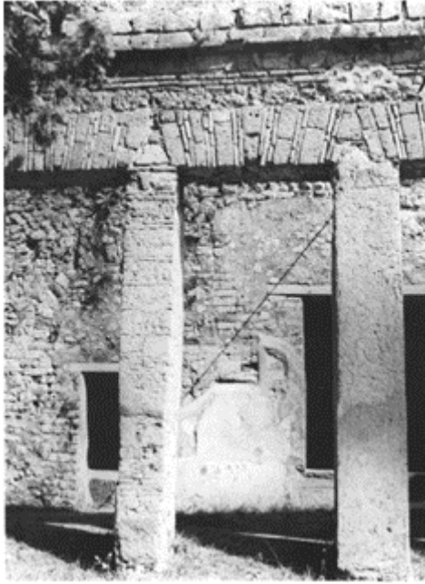
414 Openings in a portico of masonry pillars and lintel of mixed construction which are not relieved. Pompeii, Villa of Diomedes, after 62.
