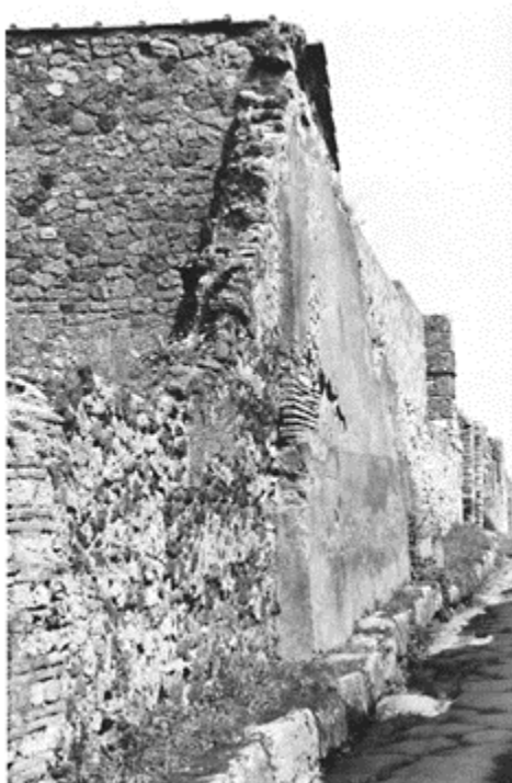
360 Pompeii, buttress-wall of brick and rubble stones, applied to a damaged building (Pompeii, VI, 2, 4).
