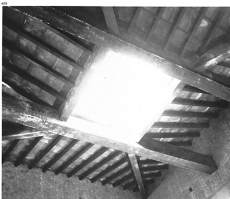
489 Reconstructed roof timbering of the atrium of the 'Tuscan' type according to Vitruvius (VI, 3, 1–6), in a domus at Herculaneum. Two main beams support the rising pieces, called the 'valley rafters', from each corner. The tiles are laid directly on the two cross-members of the compluvium and the rafters in this reconstruction. House of the Wooden Partition.
