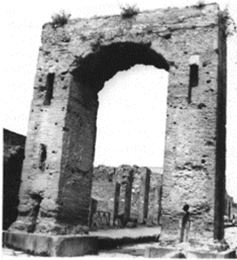
590 The Arch of Caligula at one end of the via di Mercurio at Pompeii. The structure served as a secondary water-tower, the lead pipes being housed in conduits made in the masonry piers. Two fountains, demolished in 62, were located at the foot of it.
