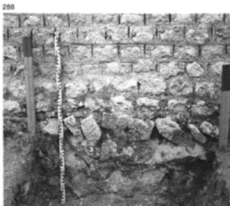
288 Foundations of a masonry wall from the Theatre of Argentomagus (St- Marcel, Indre).
