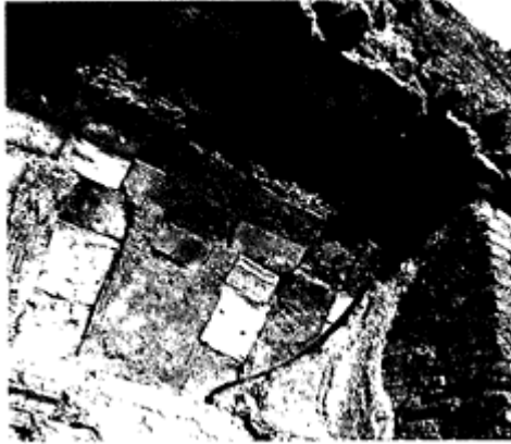
427 The intrados of an arch showing the arrangement of the bricks placed directly on to the centring. Villa dei Quintilii; c. 150.
