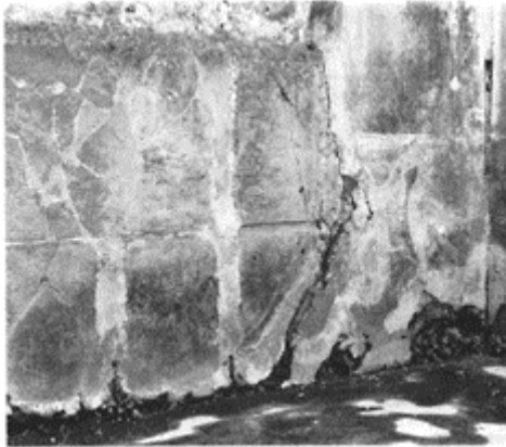
515 House of the Faun at Pompeii. Insulating wall covering made of tegulae . Size of the tiles: 64×48cm.
