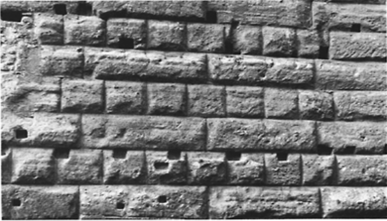
251 Detail of the wall of the Forum of Augustus showing the alternation of courses of stretchers and courses of headers.
