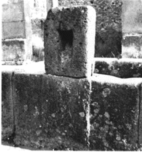
597 Pompeii: a fountain on the Via dell'Abbondanza (VII, 14). As the back edge stone has disappeared, the hole through which the supply pipe passed is visible.
