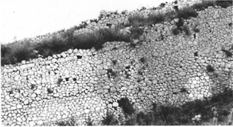
297 Walls of Terracina (between 90 and 82BC). A wall of opus caementicium , faced with opus incertum , showing the lines where the shuttering stopped.
