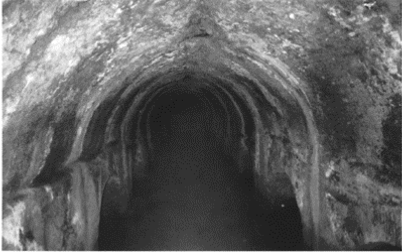
576 One of the five chambers of the large cistern of Albano, called 'il Cisternone', built in the Severan period and still in service today supplying the town. Capacity: 10,132\text{m}^3 .
