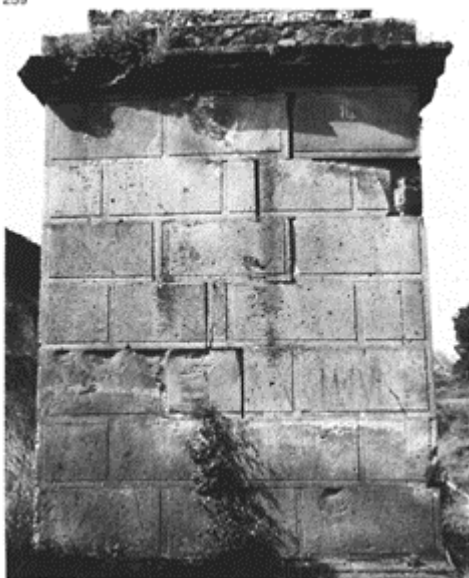
259 Actual and imitation joints in a regular facing of a funerary monument at Pompeii; necropolis of the Nuceria Gate.
