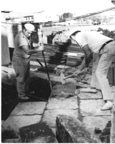
539 Laying a road surface of lava flagstones at Scafati (near Pompeii) on a bed of sand. October 1981.
