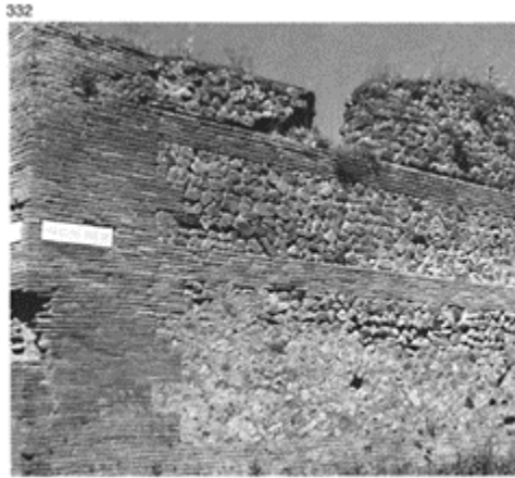
332 Opus mixtum from the last phase at Pompeii (62–79) made up of opus incertum with courses and quoins of brick (VI, 10, 15).
