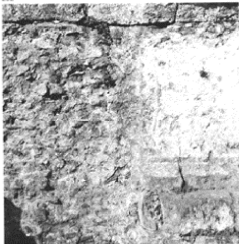
292 Opus caementicium rendered with white stucco (surviving on the right) on the podium of the Temple of Jupiter at Pompeii. Second half of the second century BC.
