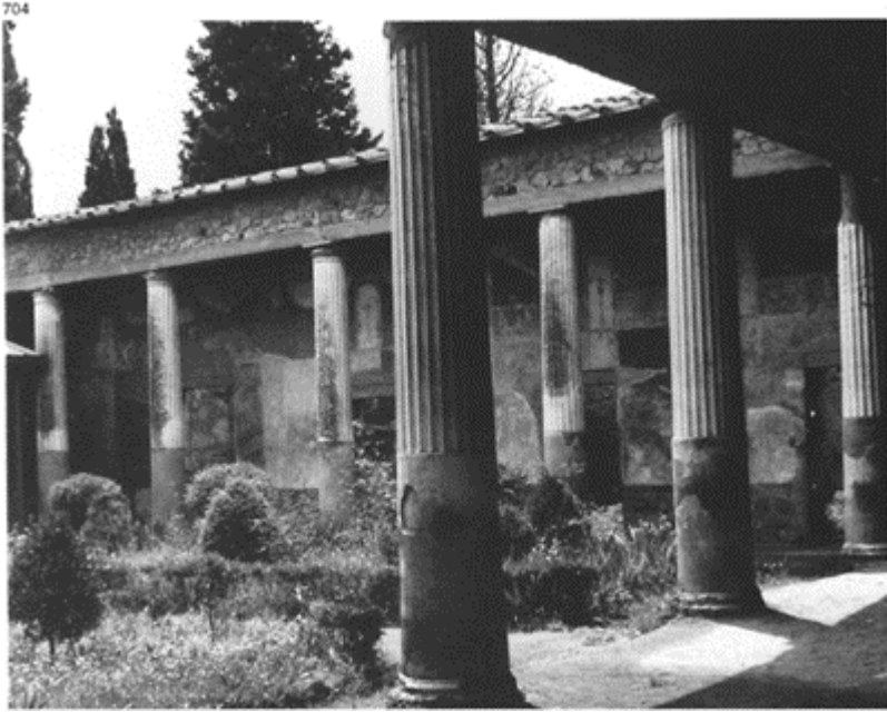
704 Peristyle in the House of Venus in the Shell (II, 3). The lowest third of the stuccoed fluted columns is protected by a covering painted red (sometimes black) in which cabling is sometimes scored.
