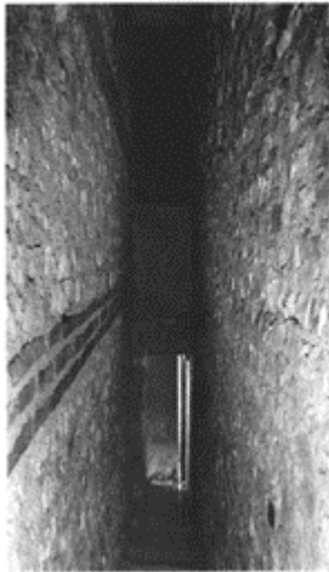
620 The narrow corridor, 4.83m high and 0.54m wide, separating the retaining wall from the building wall
