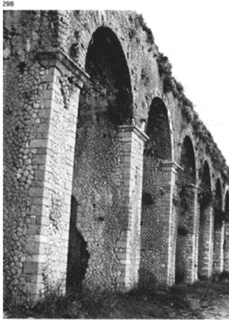
298 Supporting terrace from the Temple of Jupiter Anxur at Terracina (c. 90BC) with a facing of opus incertum with regular quoins.
