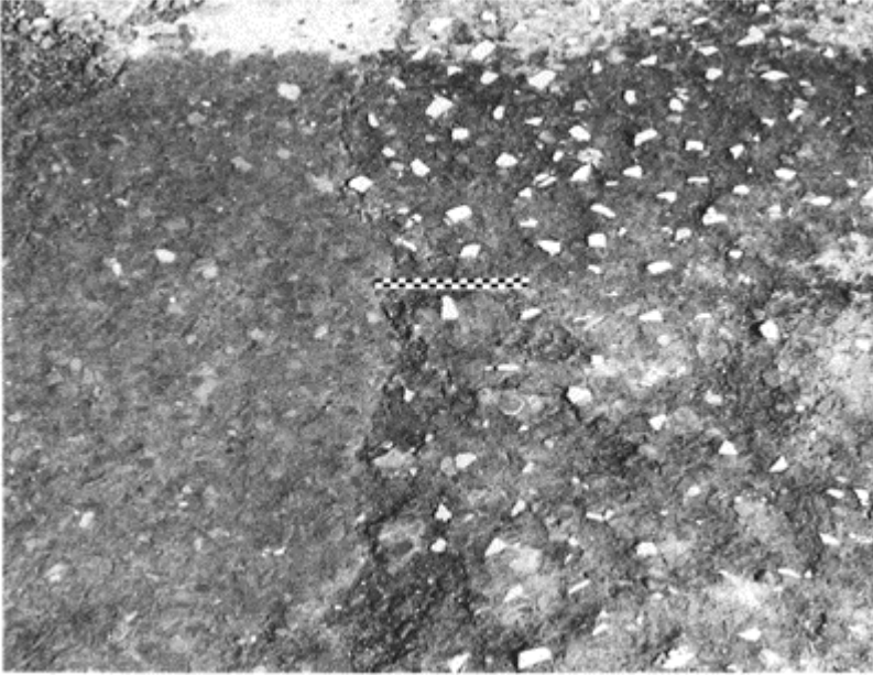
542 Pavement surface at Pompeii made of concrete with large ceramic fragments, dotted with white tessellae on the surface forming opus signinum (the Italian ‘coccio pesto’). Via di Porta Marina.
