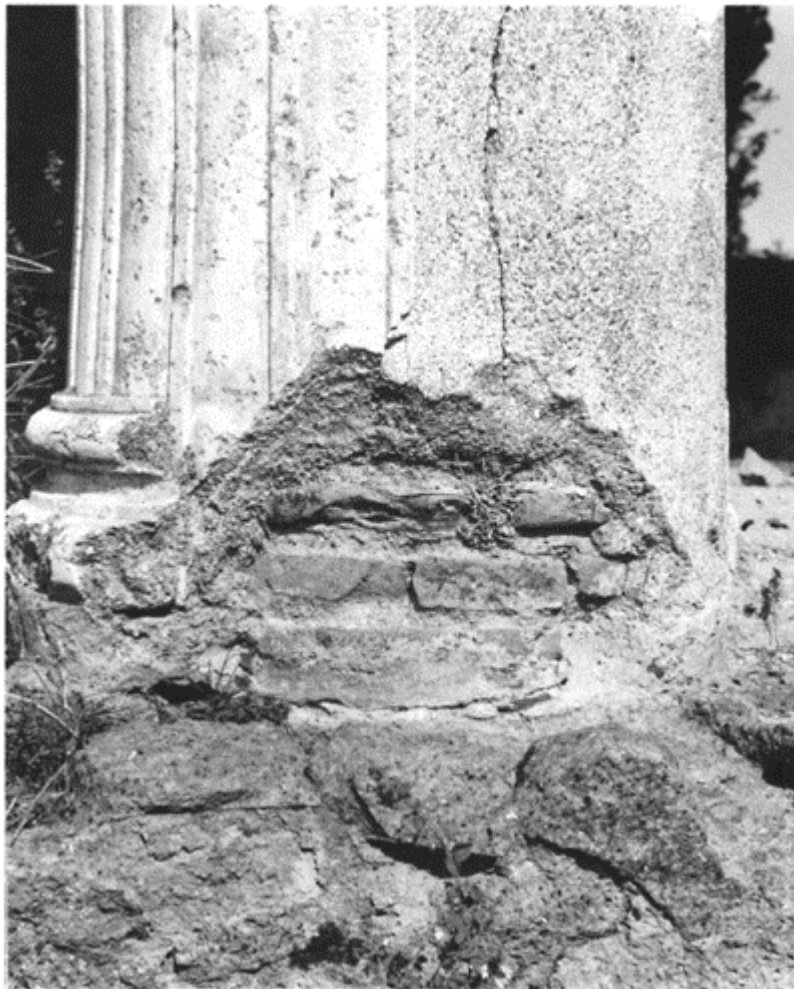
367 A masonry column of the Great Palaestra , Pompeii, fixed into place with a layer of lead (visible at the level of the scotia ) after the earthquake of 62.
