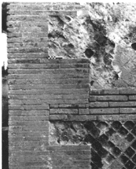
349 Quoin of finely constructed brick in a reticulate wall, with a less carefully executed horizontal course.
