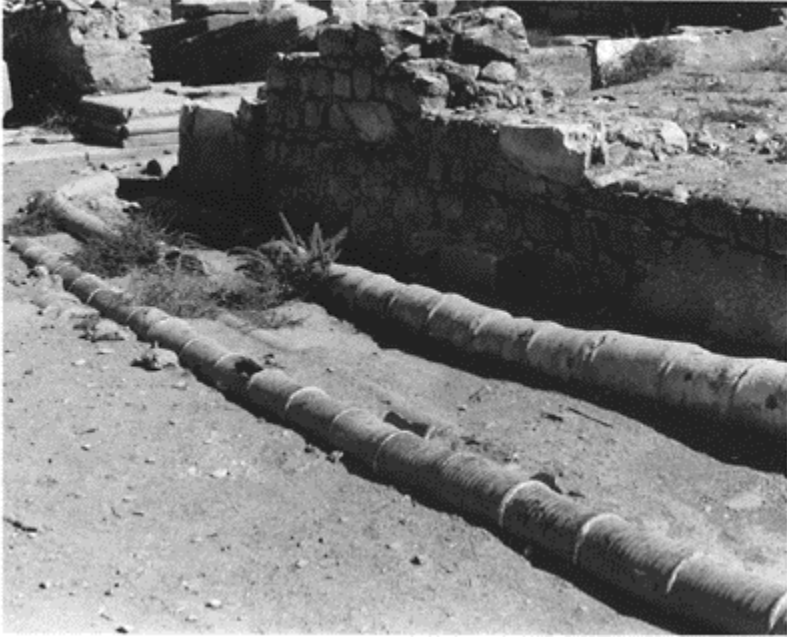
587 Pipes made of terracotta tubes jointed and sealed with lime mortar at Ephesus.
