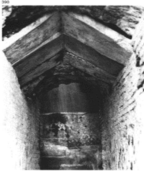
390 A gallery covered with tegulae arranged in gable-roof form; in this way a permanent coffering was achieved for corbelled masonry. Baths of Venus at Baia. Width of the passage: 90cm.
