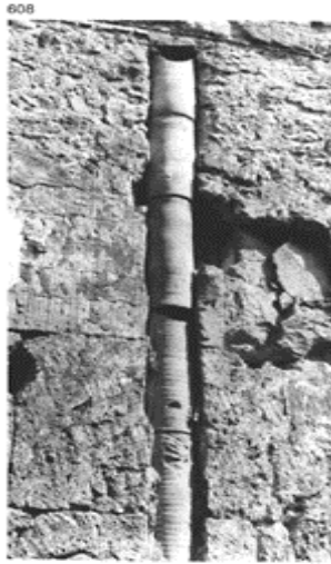
608 Drainpipes made of terracotta were protected by being sunk into a vertical groove so that they did not project from the wall. Pompeii, I, 3, 1.
