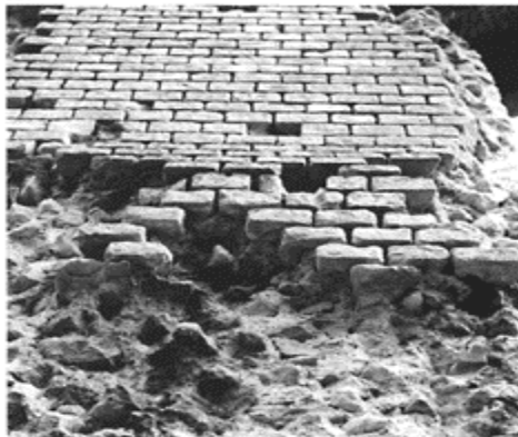
324 Aqueduct of Metz at Jouyaux-Arches (end of the first century) with very fine, regular 'petit appareil' facing with crossed joints. Notice the maizecorn outline of the rubble stones going into the infill.
